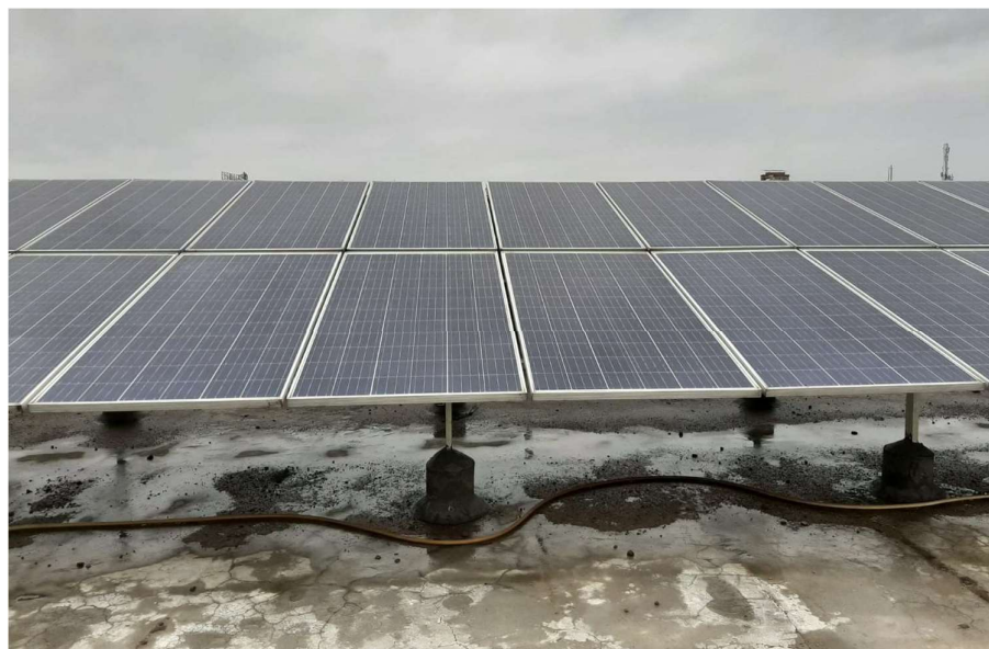
10KWp PV ROOFTOP SOLAR SYSTEM INSTALLED
